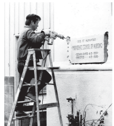
Removing cornerstone for the School of Nursing at Providence Oakland prior to demolition (1975)
